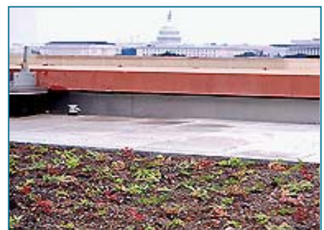
The US Department of Transportation's 68,000 sf green roof, with Capitol in background (Chesapeake Bay Foundation)
